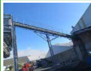
New Wet Ash System installed at Oranjevis
