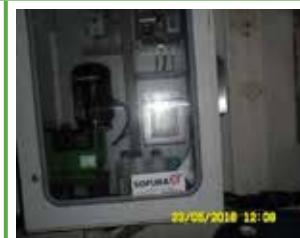
H 2 S Continuous Emission Monitor at the Chemical Scrubber at Lucky Star
